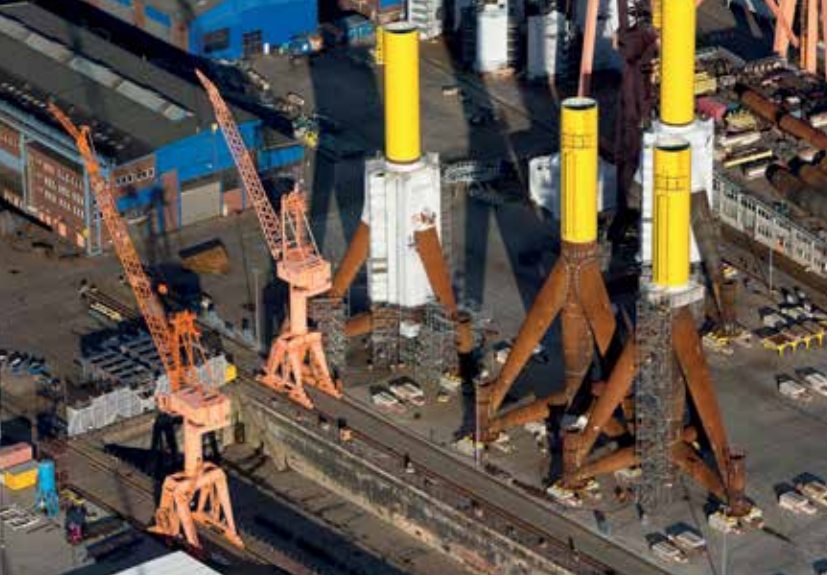
Fabrication of giant sea bed foundation supports for off shore wind turbines. Emden Stadt, Lower Saxony, Germany
